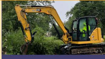
HURRICANE HELENE CLEANUP
